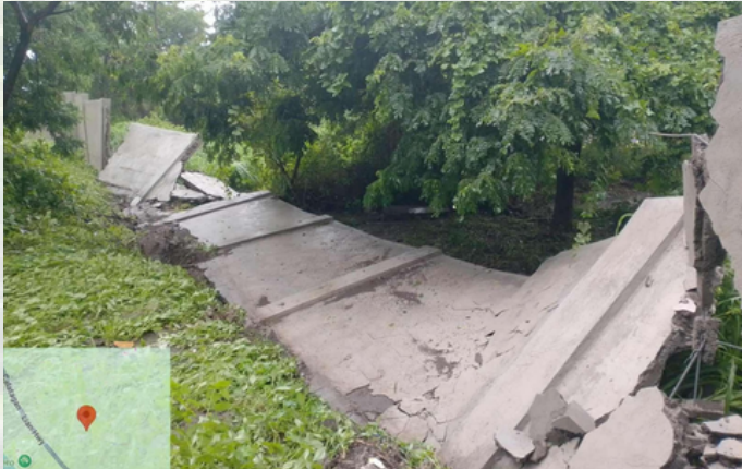
Damaged Fence, Phase 3 during Typhoon Crising, 2025
