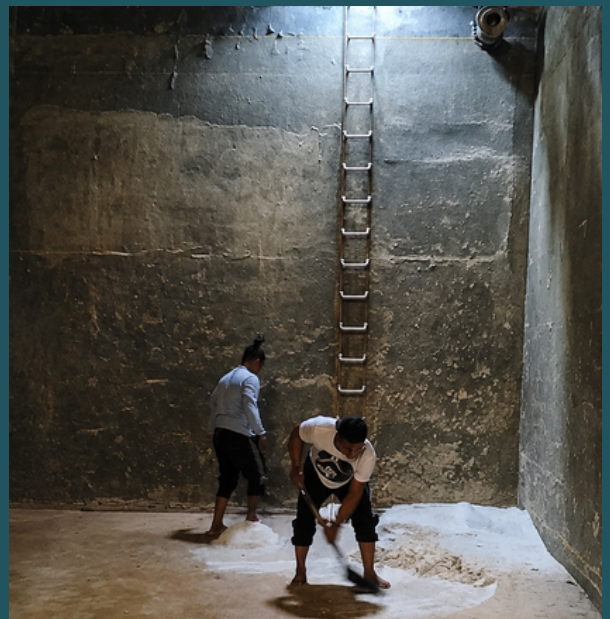
Annual Water Reservoir Cleaning
